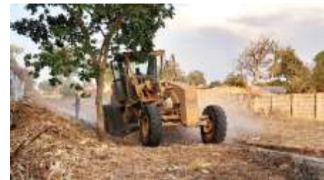
Praise the Lord that the Mufulira Road is being worked on and so is our driveway
